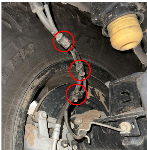
Old brake-line clips to be removed
